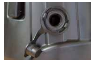
C-pipe connection for wastewater
